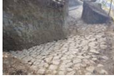
At SB 19, worn-out tiles
