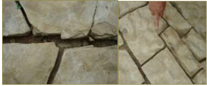
AT SB1 DETAILS SHOWING THAT THE TILES WERE CAREFULLY SET TO FIT.
